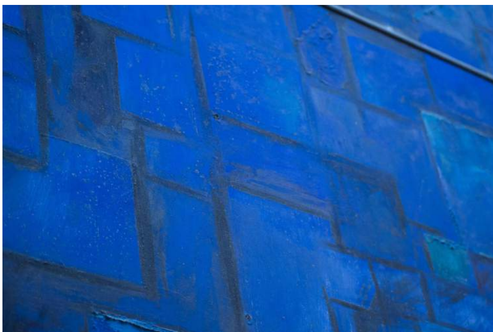
figure 23: detail paint condition demonstrating surface spotting. Photo taken by Eleanor Vallier.
